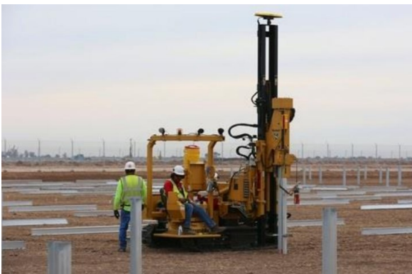
Figure 1 – Hemisphere's heading solution at work (top center), precisely aligning piles for a solar farm installation
